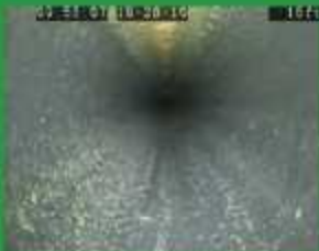
Same branch line at 16ft with no corrosion, water filled with no air-water interface
