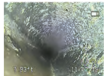
Zone 10: 3" Main – Original Galvanized Pipe over Chiller Room B
