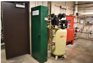
Nitrogen Generator installed in Riser Room
