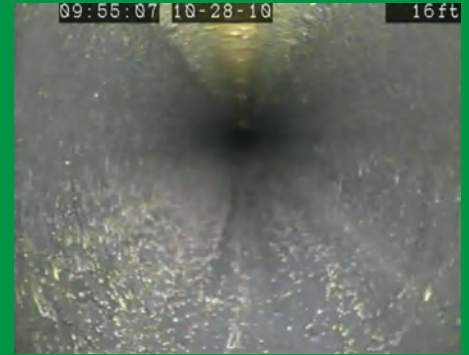
Same branch line at 16ft with no corrosion, water filled with no air-water interface
